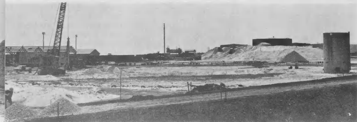
re is a section of the Lower Yard Storage Area where six new tanks of 400,000-barrels are now being erected.
